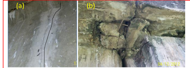
Figure 10. Visual condition of a deteriorated bridge. (a) side-view of post-tensioned beam; (b) local damage at beam joint. Source: Own elaboration
